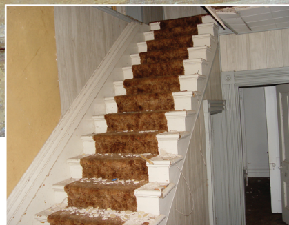
Central stairs with the bannister vandalized.
